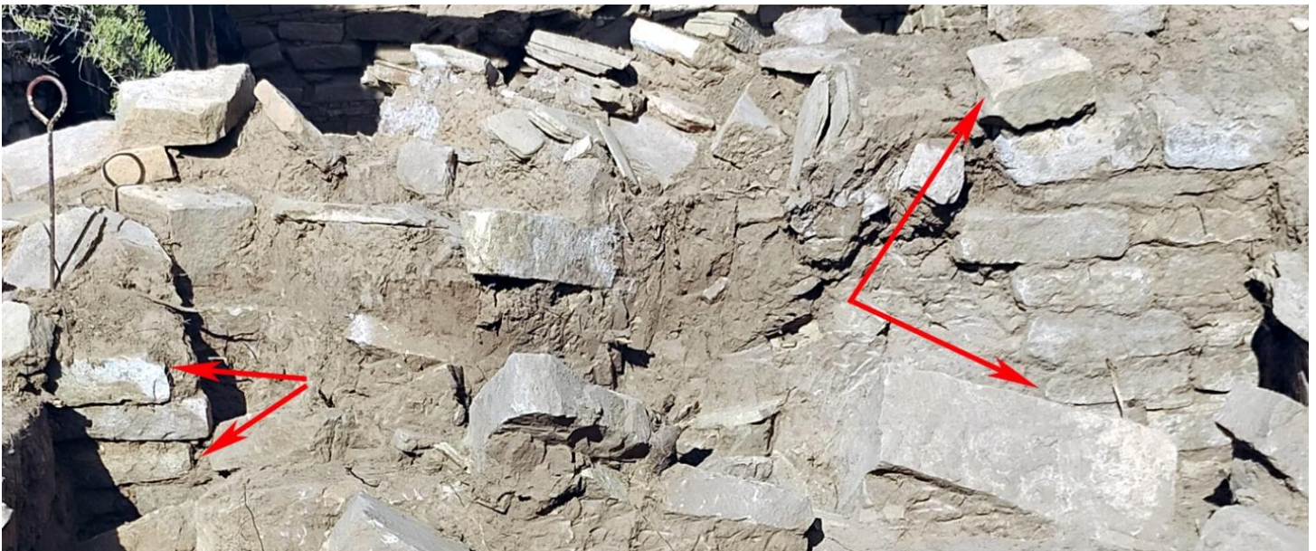
Figure 3: Profile view of the exposed exterior face of the south wall of Structure 53. Red arrows identify intact standing wall segments that bracket subsided wall stones above Other Wall Opening Feature 5.
